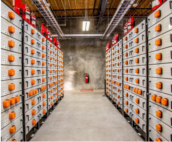
Grid Scale Energy Storage
