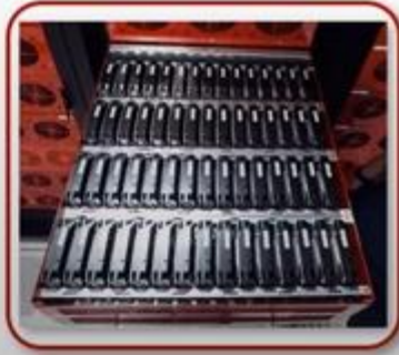
Data Center Server
